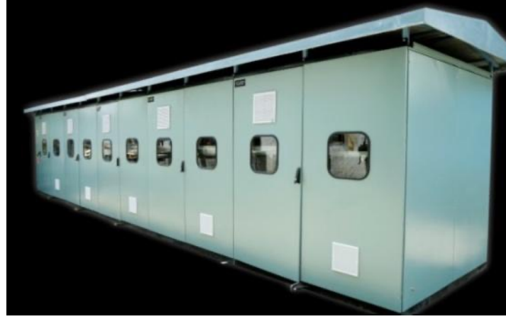
36MVAR, 11KV Auto Switched Capacitor Banks
